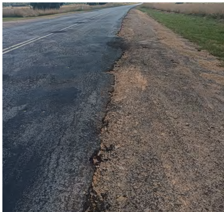
Figure 6. Poor condition of road shown opposite entrance to the site with broken edges and pot hole repair
