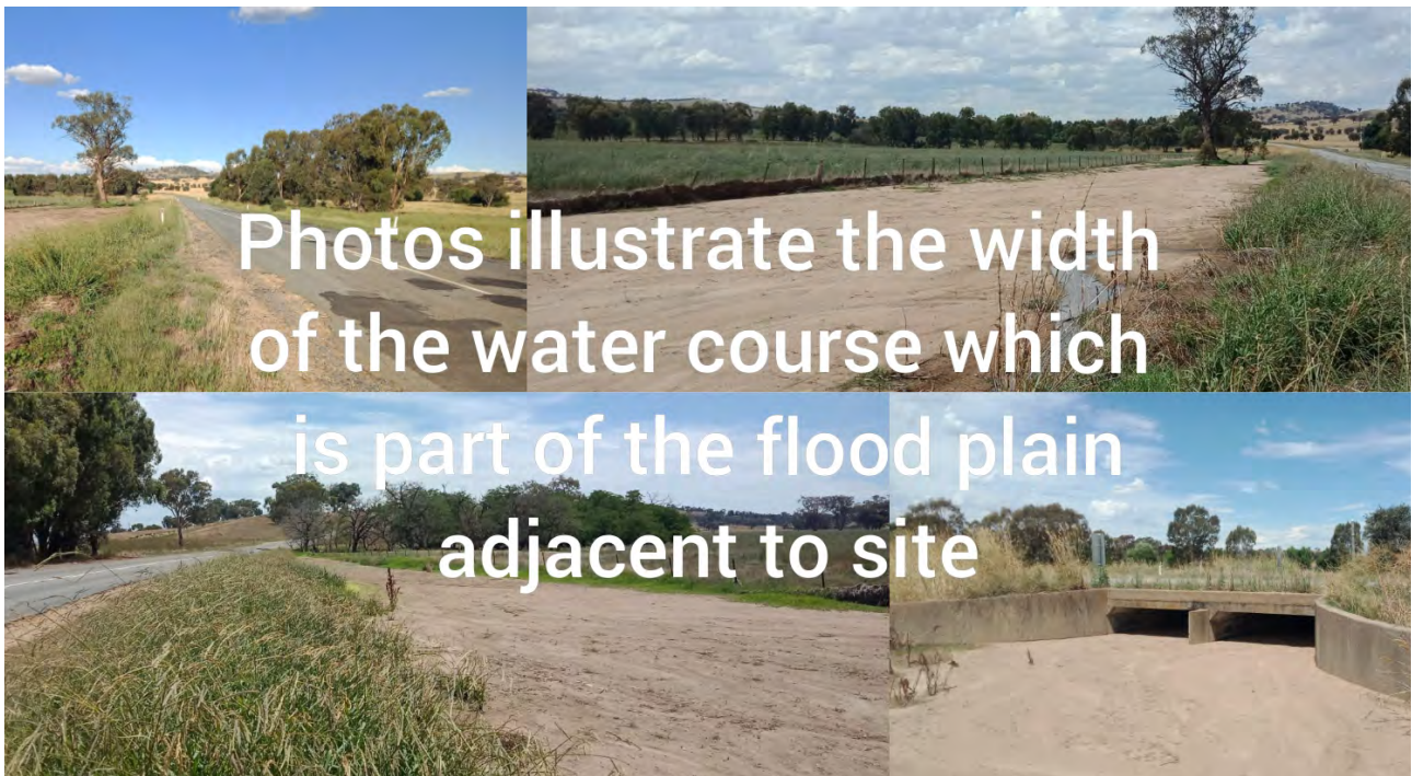
Figure 5. Oura Road looking east (top left) showing the road and drain prior to the culvert (bottom right). The culvert takes water from the north side of the road to the south side and is 140m before the Oura Station entrance (referenced in image 1). The road is subject to flooding as shown by the silt/sand build up filling the road drain (top right, bottom left). The road is narrow and does not enable safe overtaking of turning vehicles entering or exiting the site. Both sides of the road are sloping with soft soil preventing safe passing off the road surface to avoid a collision with a turning vehicle or one stopped waiting to turn.
